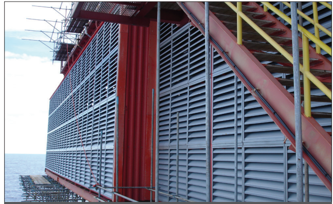
Tuff Span Louvers & Windwall Panels at offshore platform.
