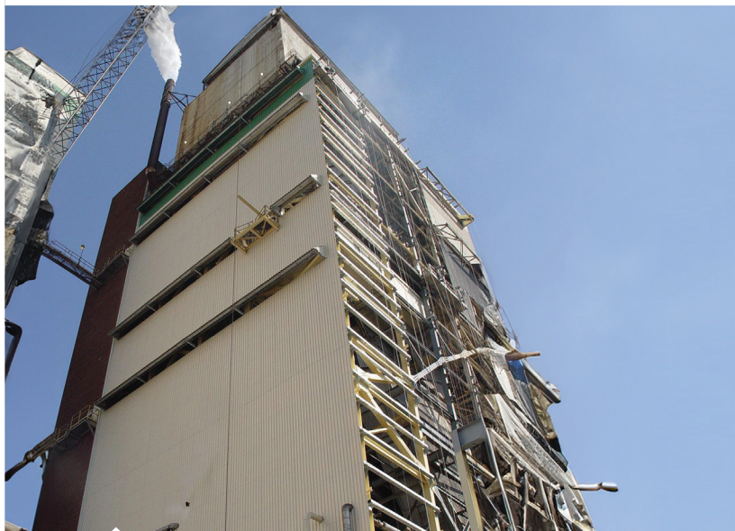
Tuff Span FM siding on 130 foot tall recovery boiler at coastal location
