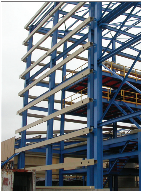
Tuff Span 8F6 girts on a chlor-alkali facility.
