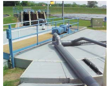
SureGrip beam-supported cover - 31' diameter Grit Basin
