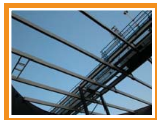
Enduro FRP structural members at a water treatment plant
