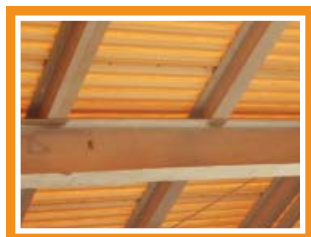
Enduro FRP primary & secondary beams
